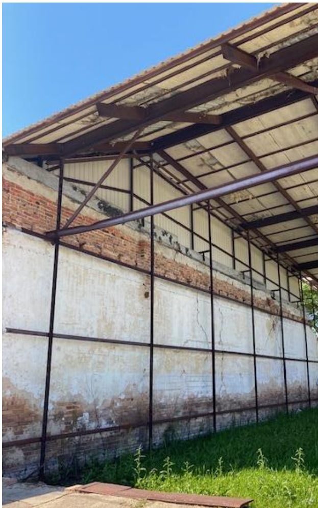
Figure #19. Close up of the side of the shopping center. Part of the brick is crumbling and cracks go through the side of the building. April 10 th , 2020.
